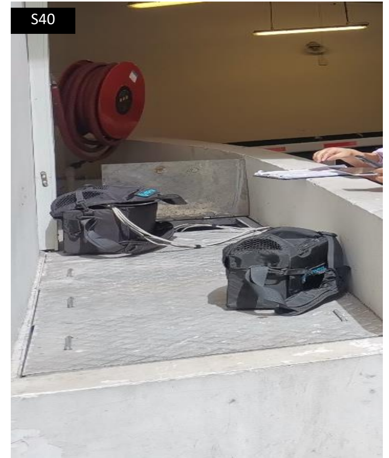
Unblock, Open space, meter in metal and concrete chamber
